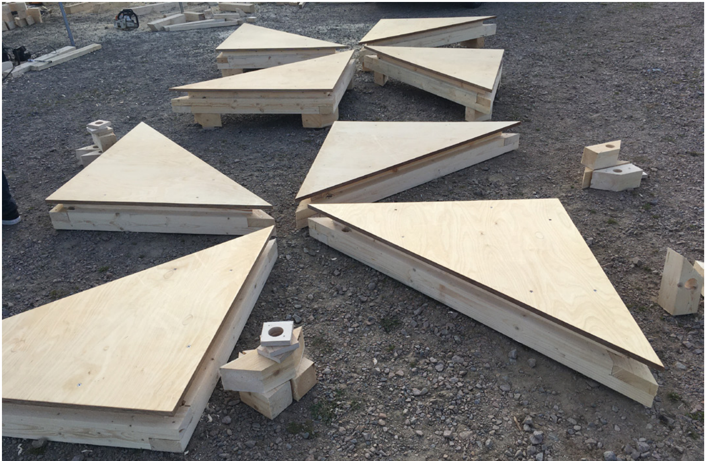
The dance floor is both modular and movable. Pictured here under construction 5th September, 2020. Photo by Anna Asplind
